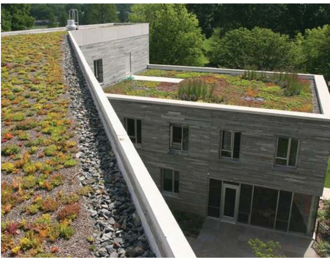
Green roofs are increasingly popular on college campuses. This dormitory at Swarthmore College has green roofs on two levels, one of which is visible from inside the building.
