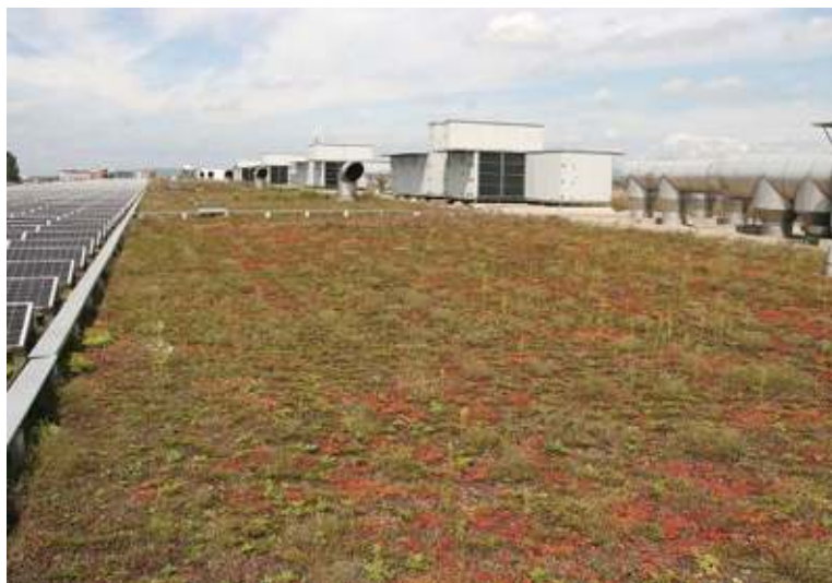
Extensive green roofs, especially when installed on a wide scale, provide a range of benefits including stormwater management.
