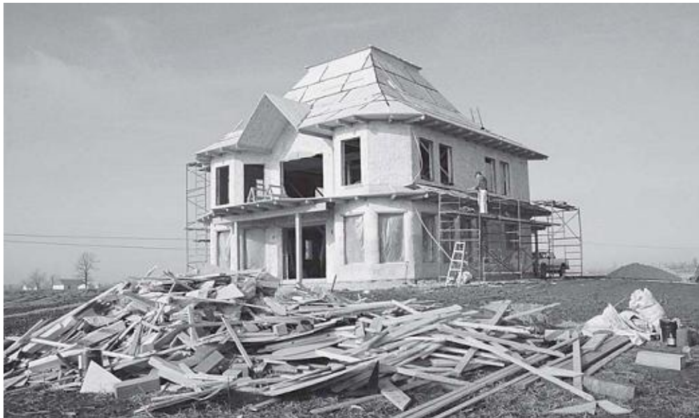
A small pile of recyclable materials is often all that is left over after construction of a straw bale house.
