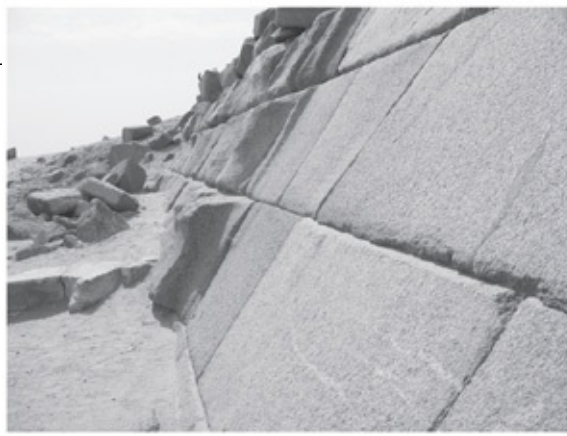
Fig. 1.2. Not all casing stones of the third pyramid were cut smooth. Granite may have been chosen for its durability as opposed to its beauty.
